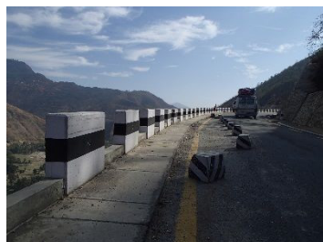
Present condition of damaged road of Station 15+520
