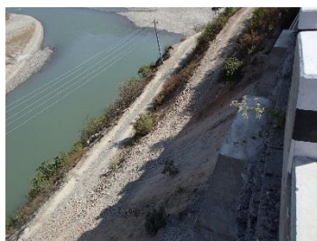
Unpaved road and utility pole lie below Station 11+620
