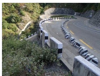
Present condition of damaged road of Station 33+695
