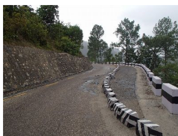
Present condition 2 of damaged road of Station 33+440
