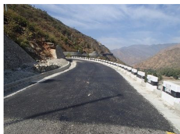
Present condition of damaged Road of Station 11+620
