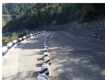
Present condition 1 of damaged road of Station 33+440
