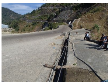
Water Pipes from the Surrounding Mountain (Set up by DOR)
