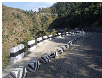
Surrounding 2 of damaged road Station 33+440 (Distant View)
