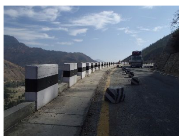
Present Condition of Damaged Road of Station 15+520
