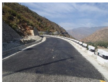
Present Condition of Damaged Road of Station 11+620
