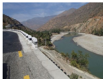
No Settelement along Sunkoshi River lie below Station 11+620
