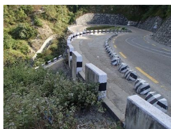
Present Condition of Damaged Road of Station 33+695
