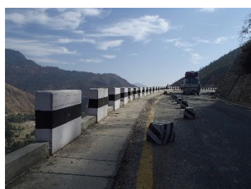
Present Condition of Damaged Road of Station 15+520
