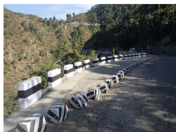
Surrounding 2 of Damaged Road Station 33+440 (Distant View)
