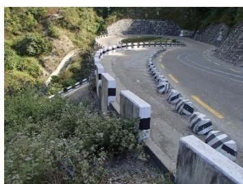
Present Condition of Damaged Road of Station 33+695
