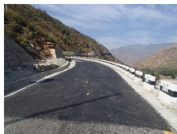
Present Condition of Damaged Road of Station 11+620
