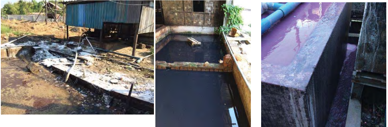
Treatment water by WWTP in some factories
