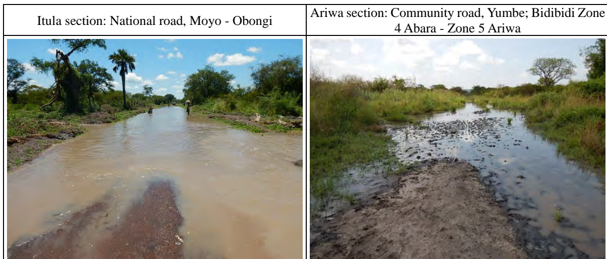
Photo 6.2-3 Flooding Situation Derived from the Deficiency of Road Surface Height
