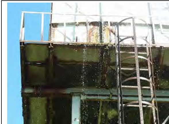
The elevated water tank of Itula Piped Water Supply System, leaking due to aging. The support structure and ladder are corroded and could collapse. (Itula Sub-County, Moyo District)
