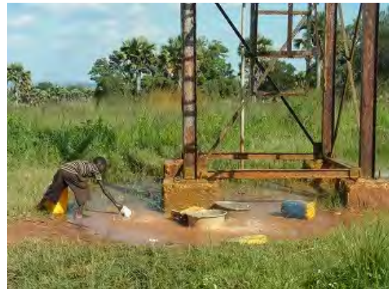
The elevated water tank of Itula Piped Water Supply System. A resident is ladling up water from a puddle of leaking water. (Itula Sub-County, Moyo District)
