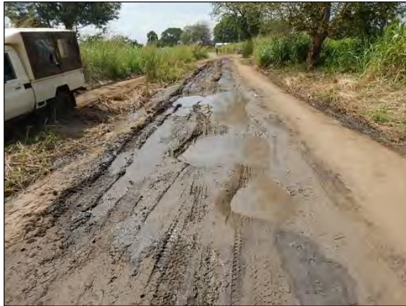
1 August 2017 Potholes due to delay of appropriate road maintenance Yumbe – Manibe (Class-B) Road
