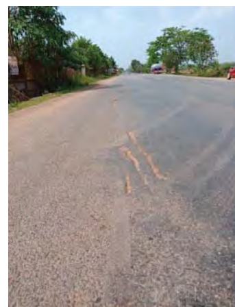
Fixed Defect (NR-13N)
