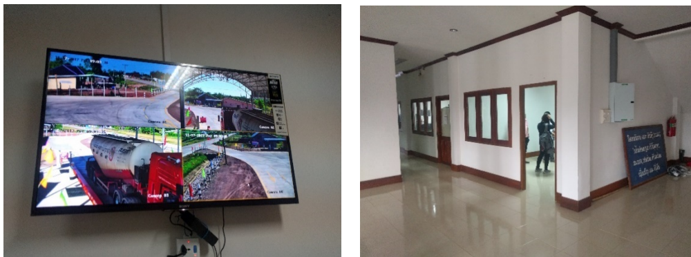
Monitor and Server Room in DPWT Savannakhet
