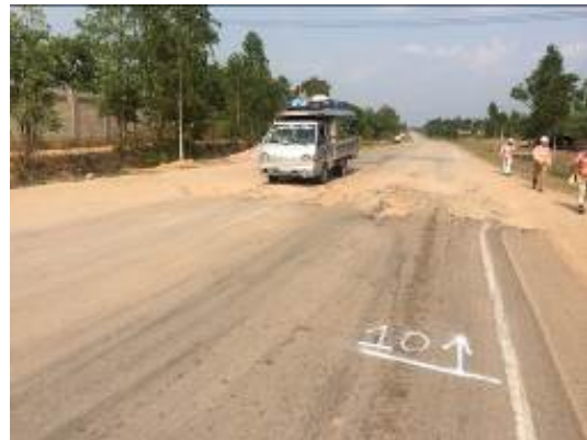
Deformation of surface
