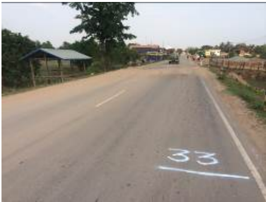
Crocodile crack and rutting development
