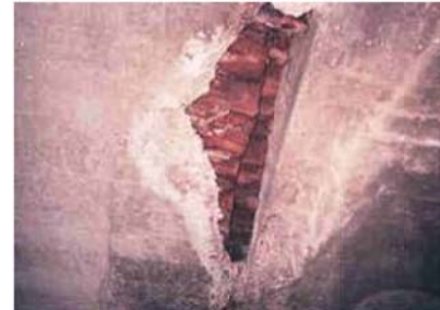
Shortage of concrete casting
