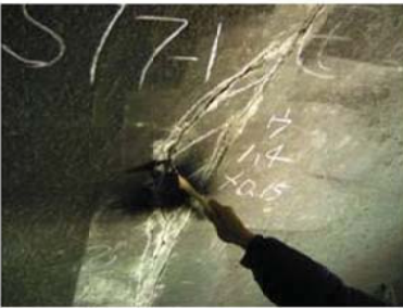
Crack by poor workmanship in setting form
