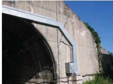
Crack on portal
