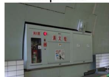
Fire extinguisher and Plug
