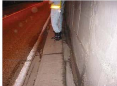
Deformed ditch in roadside
