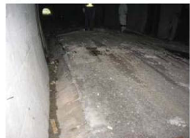
Heaving of road surface
