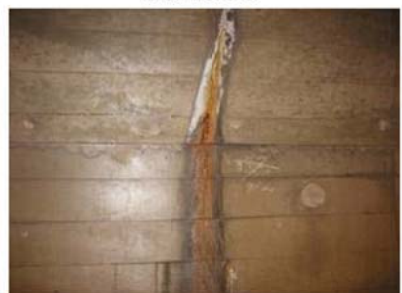
Leakage in joint
