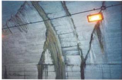
Crack on lining
