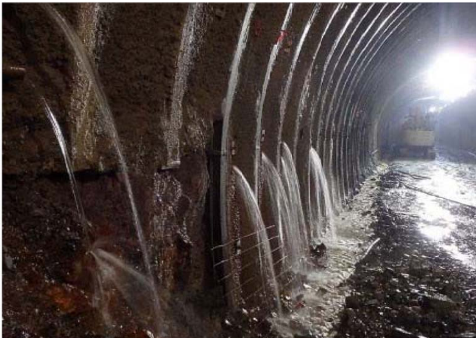
Water leaking from fault fracture zone of Mizuho tunnel
