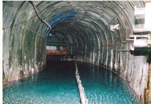
Drainage Drift of Kanmuriyama Tunnel
