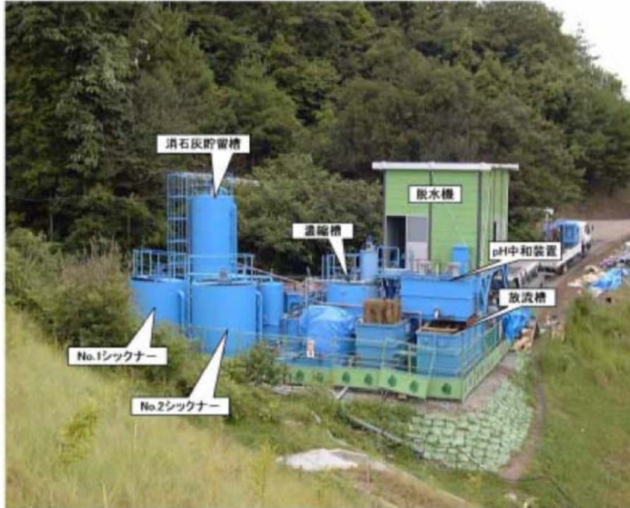
Leachate treatment plant
