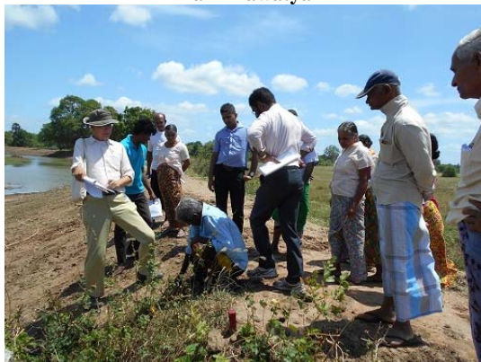
A farmer confirming a hole in the upstream surface. Study of risk of piping.
