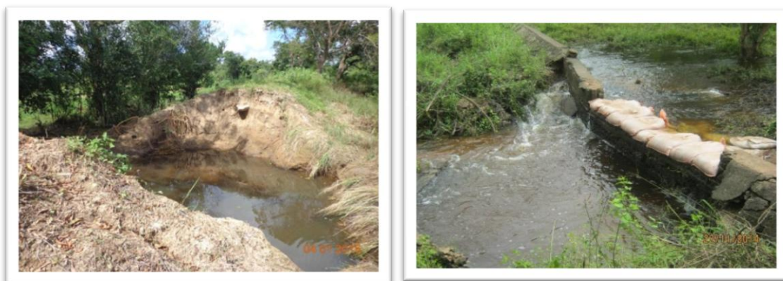
(左：堤体決壊、右：洪水吐崩壊)
