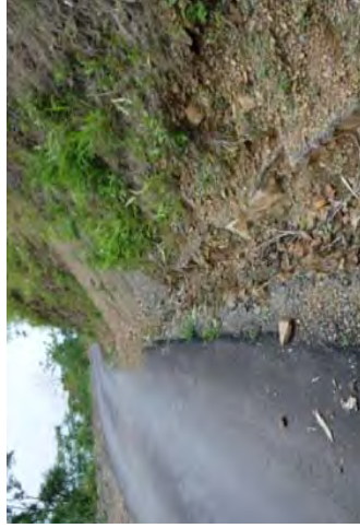
Old pavement destroyed by landslide
