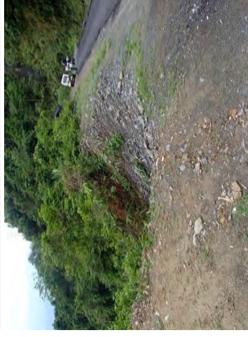
General slope of landslide
