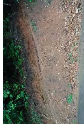
loose soil deposit
