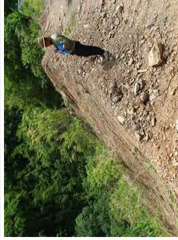
Collapse of dumped soil on valley side
