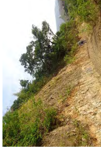
Link road on the upper landslide
