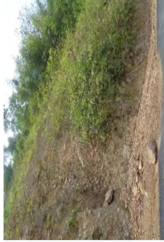
Debris accumulate at road side
