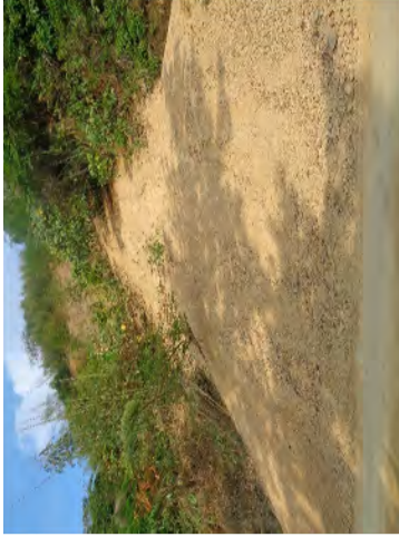
Full view of landslide
