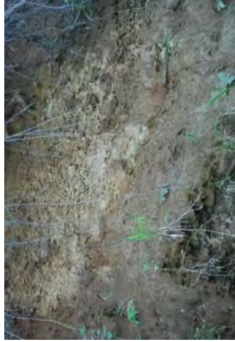
Condition of scarp portion
