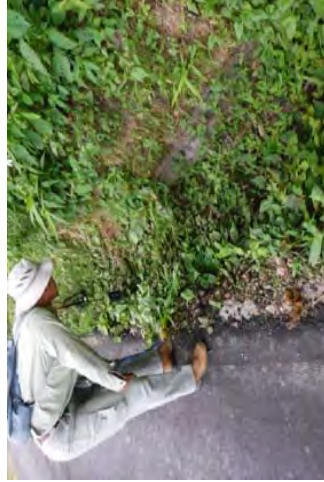
Old pavement covered by landslide
