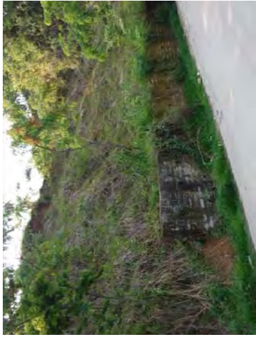
Full view of landslide
