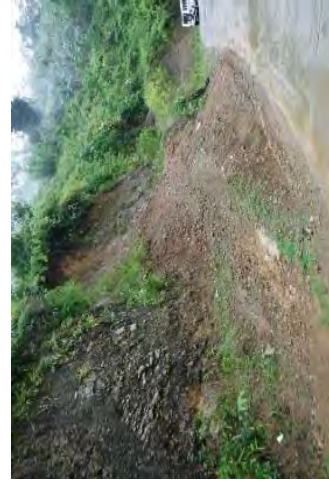
Minor landslide on earthen road
