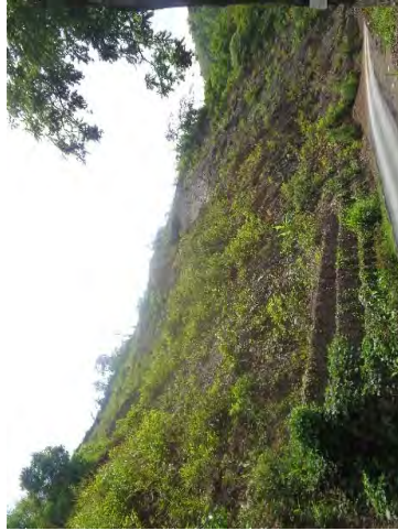
Full view of landslide
