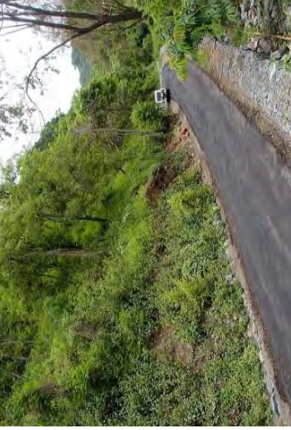
Road sinking in landslde area
