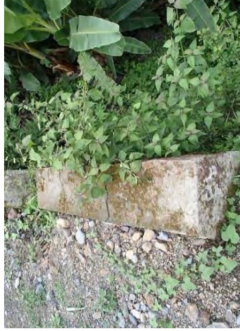
Crack on retaining wall at side of landslide
