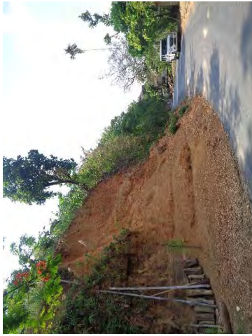
Full view of landslide
