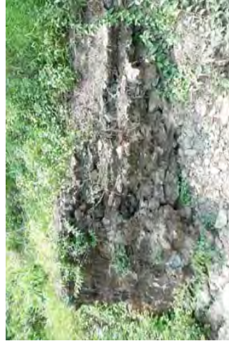
Deformation of retaining wall
