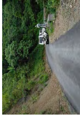
Slope of landslide
