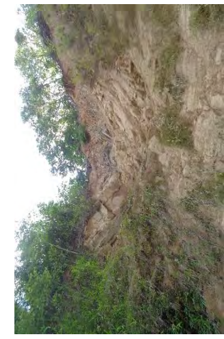
Head portion of landslide
