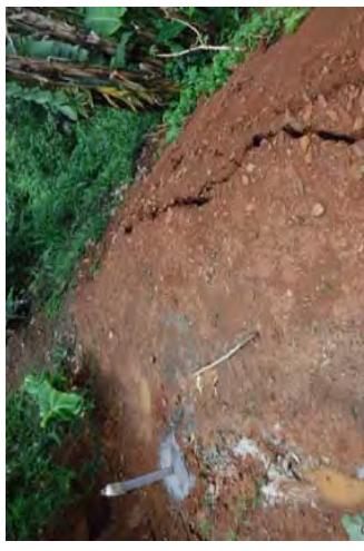
Crack of dump soil
