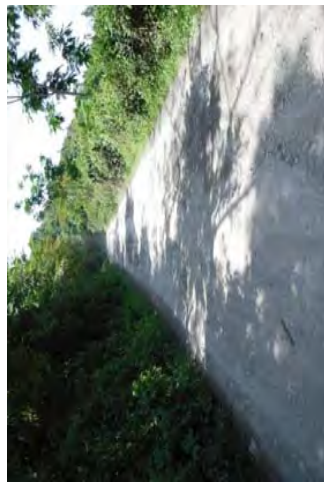
Road condition (Sinking)
