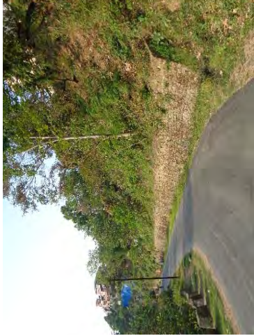
Full view of landslide
