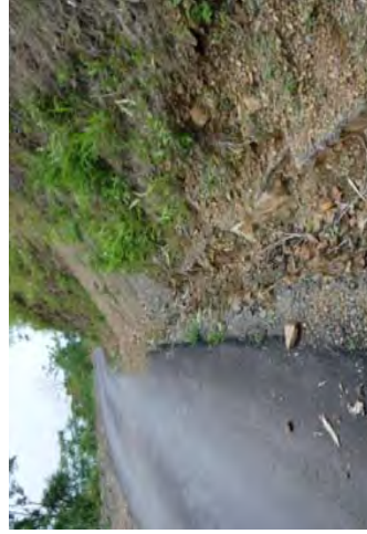
Old pavement destroyed by landslide
