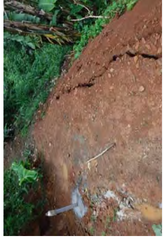
Crack of dump soil
