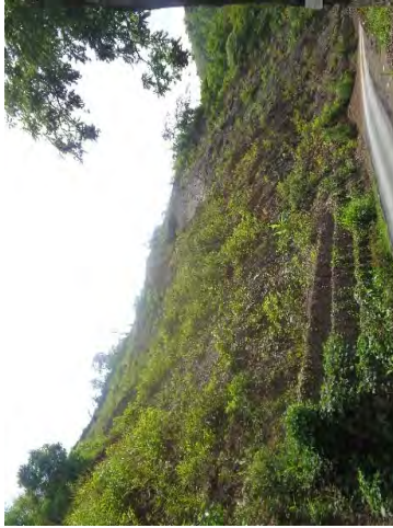
Full view of landslide
