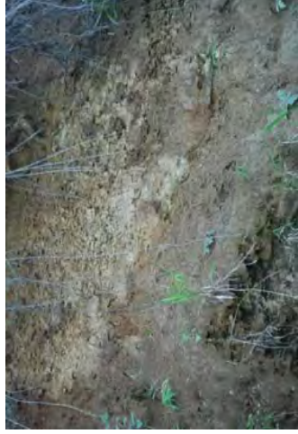
Condition of scarp portion
