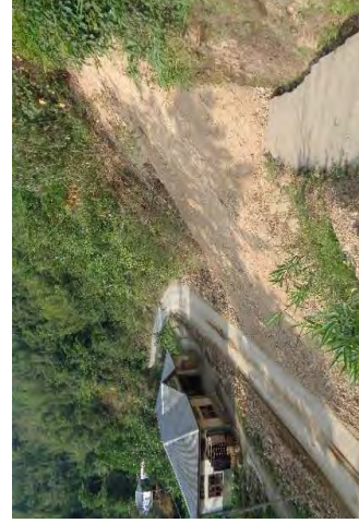
Slope of landslide
