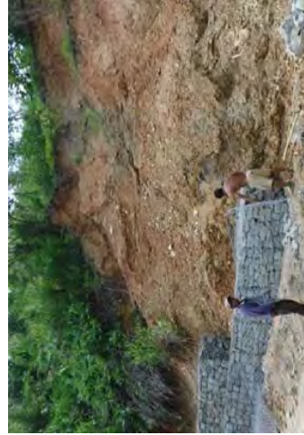
Condition of landslide
