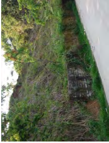
Full view of landslide
