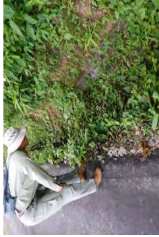
Old pavement covered by landslide
