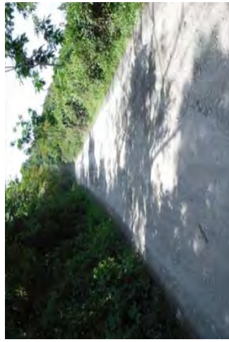
Road condition (Sinking)
