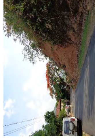
General slope of landslide
