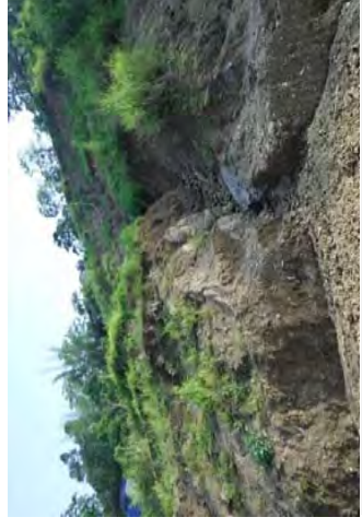
Front view of landslide
