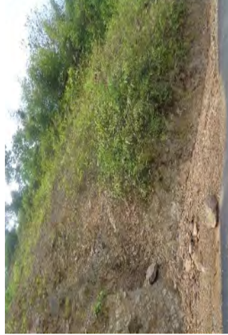
Debris accumulate at road side
