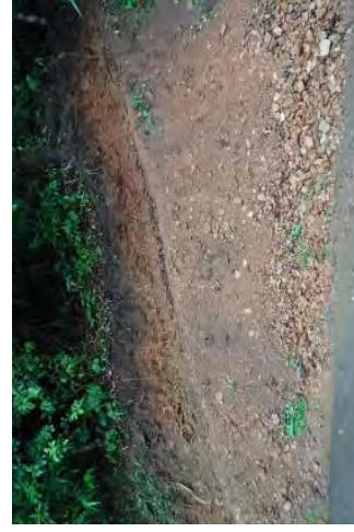
loose soil deposit
