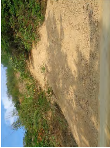
Full view of landslide
