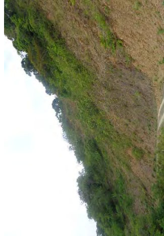
Upper link road on landslide
