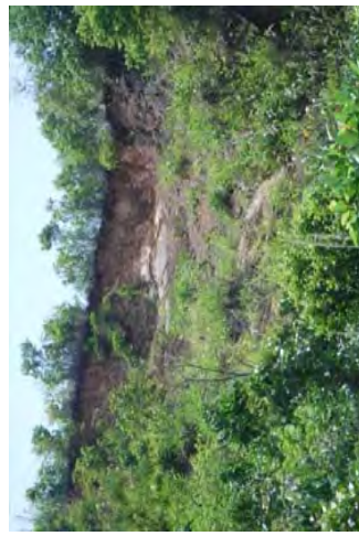
Scarp of landslide
