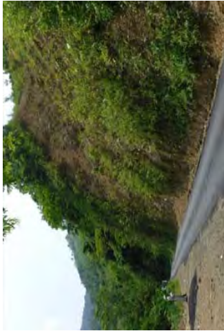
Full view of landslide
