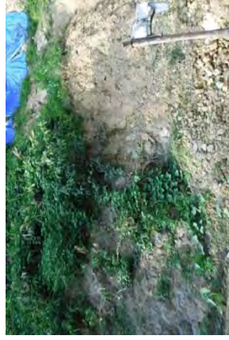
Vegetation, loose soil on hill side
