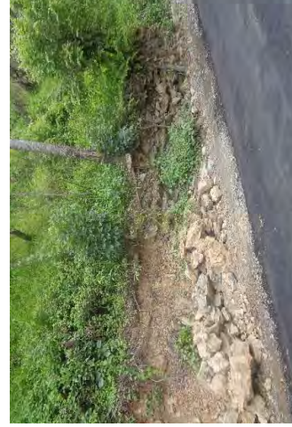
Deformation of wall
