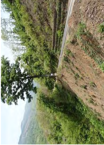
Collapse of dumped soil on valley side
