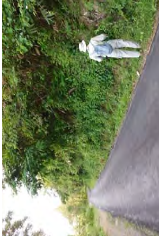
View of landslide
