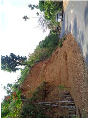
Full view of landslide
