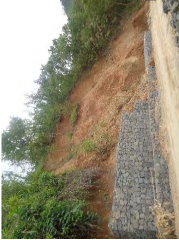
Full view of landslide
