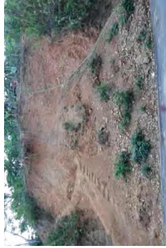
Front view of landslide
