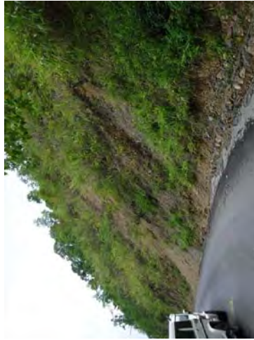
Full side view of landslide
