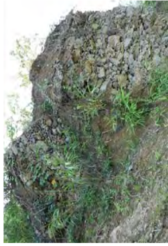
Deformation of gabion wall
