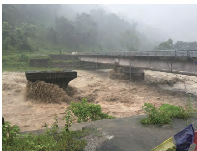
River swollen by a torrential rain and Jigmeling Bridge (left: old bridge pier, right: new bridge)
