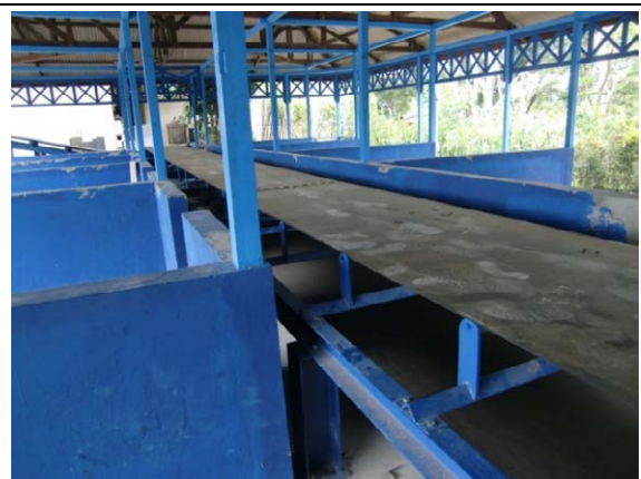
Belt Conveyor Installed in MRF
