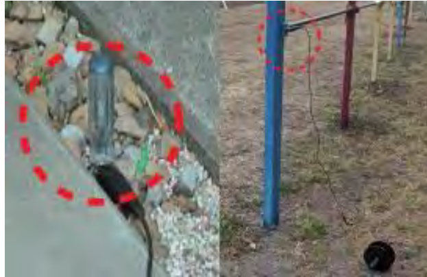
Figure 3: Place for Earthing
