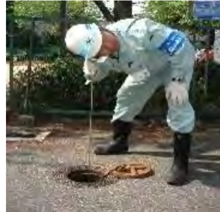
Figure 4: Detection from Valves by Acoustic rod
