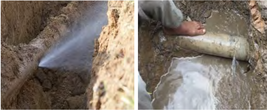
Figure 1: Water Loss from hole (left) and crack (right) of an Asbestos Cement Pipe
