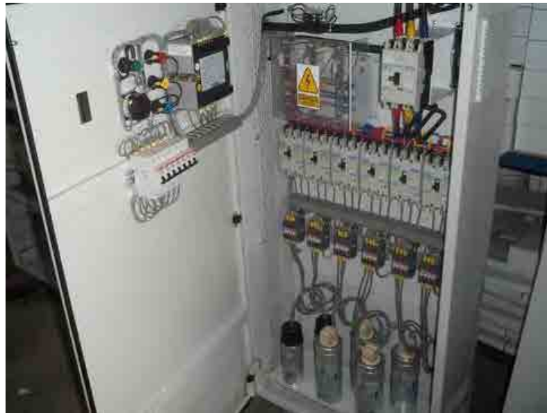
Figure 1 Capacitor bank inside electrical control pan
