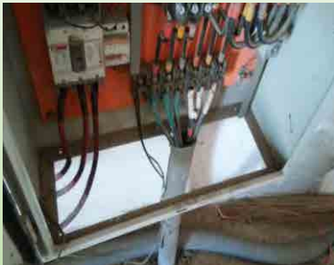
Broken base plate
