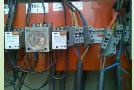
Exposed electrical parts
