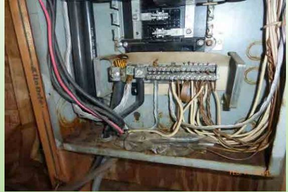
Wet & moist condition
