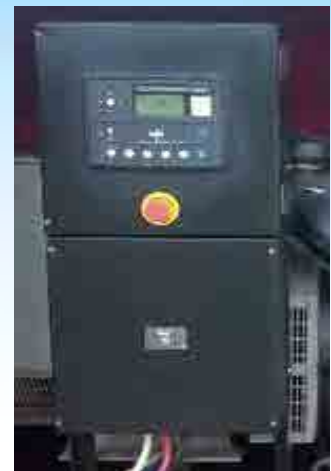
Electrical Control panel
