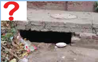
Kerb Grating Missing
