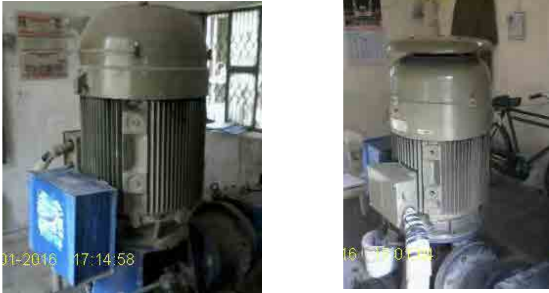
Figure 2 : Excellent Condition of Priming Box and Insulation of cable of Motor Terminal Box
