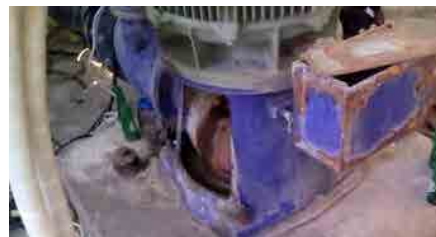
Figure 1: Poor Priming Box and Poor Cable Insulation
