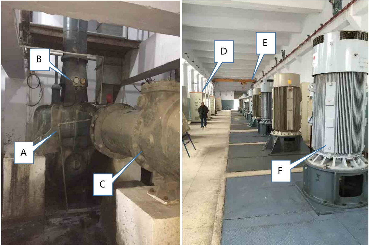
Control panel, Motor, Non return valve, Pump, Crane, Pressure gauge
