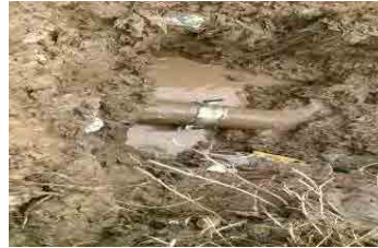
Pipe leakages causes the system to get clogged
