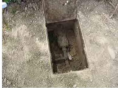
Meter almost buried in the soil
