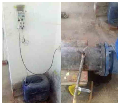
Dosing of Chlorine in WASA system
