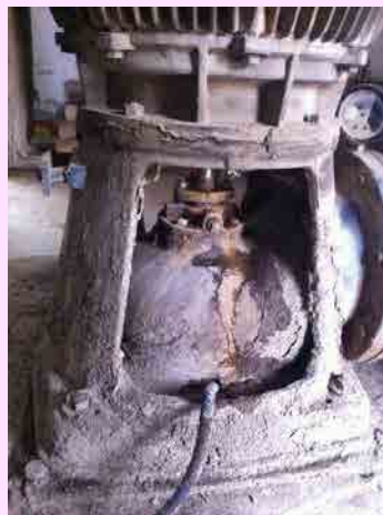
Corrosion & Contamination Leakage (slip and fall)
