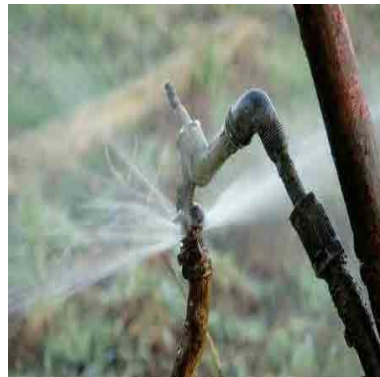
Leakages from meter connections
