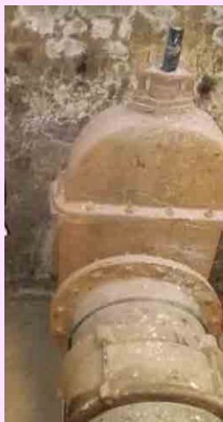
Corrosion and Contamination
