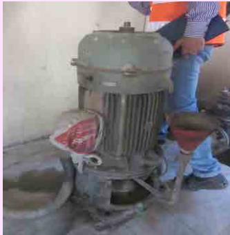
Missing Top Cover, Cut Hazard, Tool Lost and Material Damage Hazard
