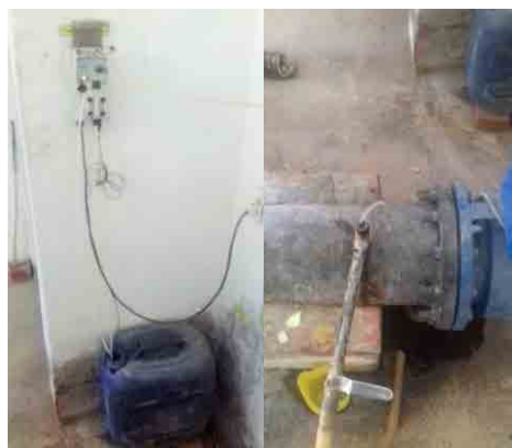
Dosing of Chlorine in WASA system
