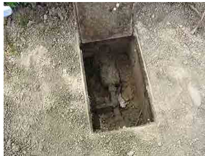
Meter almost buried in the soil
