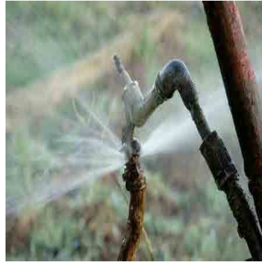
Leakages from meter connections
