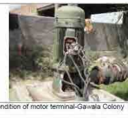
Condition of motor terminal-Gawalla Colony
