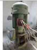
View of motor & pump-Shahdin Park
