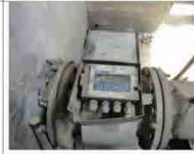
Out of order water flow meter-Maskeen Pura
