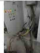
Panel and cabling condition-Shalimar Scheme
