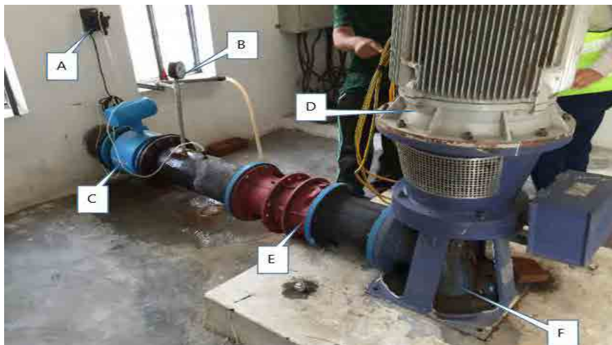
Pump, Motor, Flow meter, Non return valve, Pressure gauge, Chlorine dosing pump
