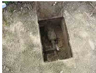
Meter almost buried in the soil
