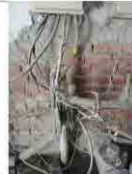
Cabling condition-Faten Garh Dispensary
