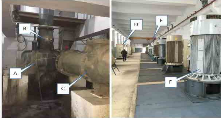
Control panel, Motor, Non return valve, Pump, Crane, Pressure gauge
