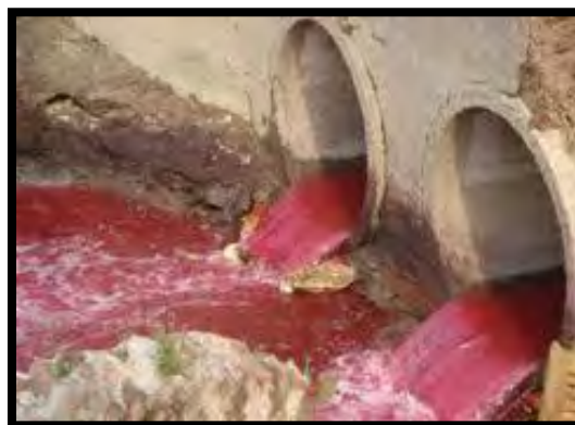
Figure 3: Observation of colored water at manhole and sewer
