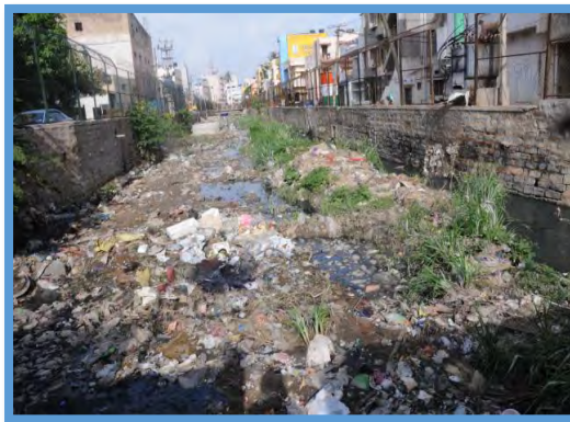
Figure 1: Encroachment around Drains
