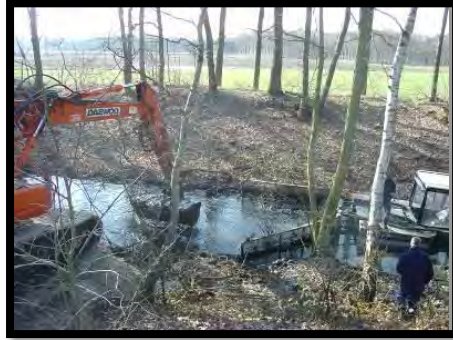
Figure 10: Damage to the Bank
