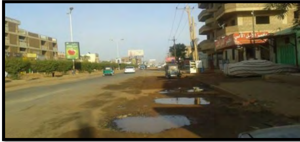
Figure 3: Ponding on the Road
