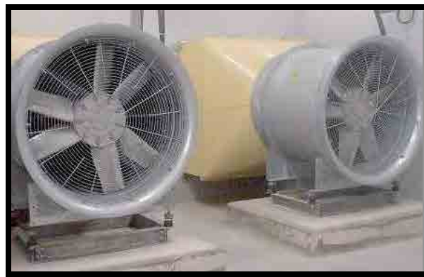
Figure 10: Exhaust Ventilation System
