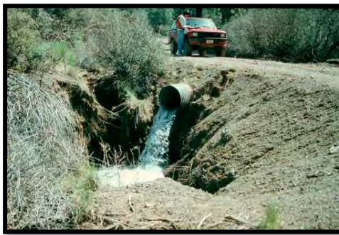
Figure 4: Erosion of Culvert Bed
