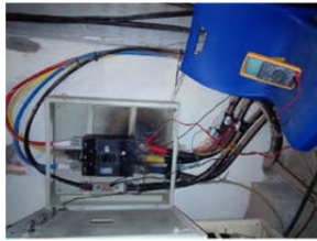
FIG.5 - MAIN GEAR SWITCH 800A AND METERING POINT. POOR CABLE TERMINATION. (Inside Equipment Room-Ground floor)
