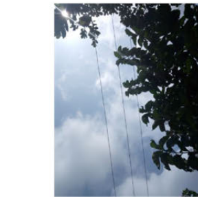
FIG. 1 – RIGHT OF WAY OF 33KV OVERHEAD LINES IMPACTED BY OVER-GROWN TREES
