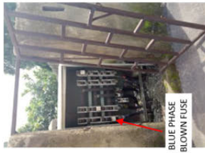
FIG. 4 – FEEDER PILLAR, GATE - BROKEN, LOW LEVEL. DOOR OPENED TO RAIN/SUN.. TOO CLOSE TO ENTRANCE.
