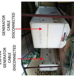
FIG.18 – GENERATOR 60KVA (Generator area)
