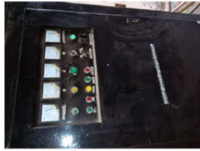
FIG.11 – CHANGEOVER PANEL. WITH AUTO AND MANUAL SWITCHING PROVISIONS. (Generator area)
