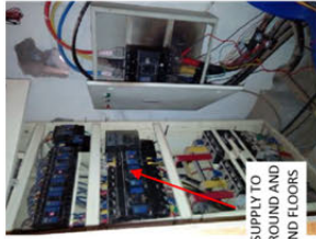
FIG.6 - MAIN GEAR SWITCH 800A AND MAIN DISTRIBUTION BOARD. (Inside Equipment Room-Ground floor)
