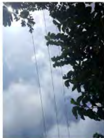
FIG. 1 - RIGHT OF WAY OF 33KV OVERHEAD LINES IMPACTED BY OVER-GROWN TREES
