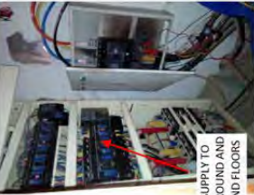
FIG. 6 - MAIN GEAR SWITCH 800A AND MAIN DISTRIBUTION BOARD. (Inside Equipment Room-Ground floor)
