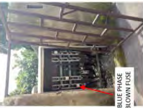
FIG. 4 - FEEDER PILLAR. GATE - BROKEN. LOW LEVEL. DOOR OPENED TO RAIN/SUN.. TOO CLOSE TO ENTRANCE.
