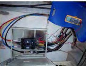
FIG. 5 - MAIN GEAR SWITCH 800A AND METERING POINT. POOR CABLE TERMINATION. (Inside Equipment Room-Ground floor)
