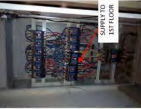
FIG. 7 - SUB MAIN DISTRIBUTION BOARD. (Inside Equipment Room-Ground floor)
