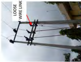
FIG. 2 - HT POLES AND 33KV OVERHEAD LINES. STANDARD FUSES ARE REMOVED. LINE 3 WIRE LINK LOOSELY CONNECTED
