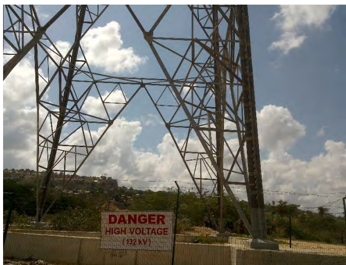
Photograph A Electricity Tower
