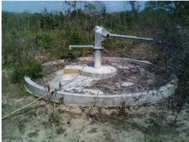
Figure 16 : Borehole equipped with hand pump (inoperative)
