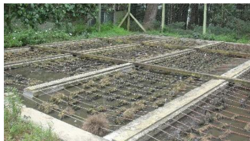
Leachate Collection and Treatment System
