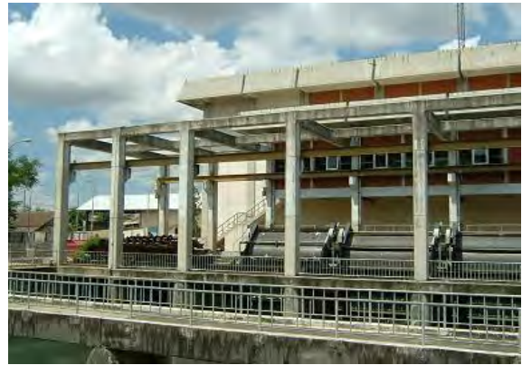
Pump station constructed at Western Canal
