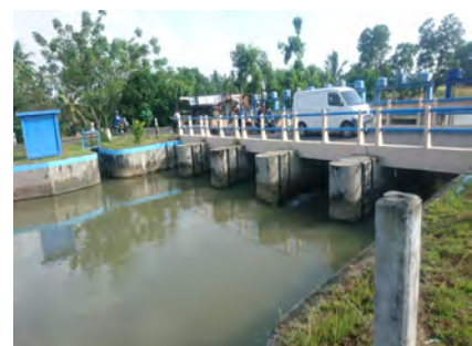
Komering irrigation facility
