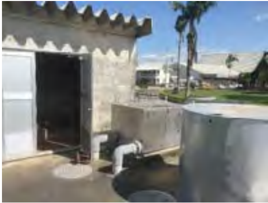
Photo 38 Screen and Entrance of Mechanical Room
