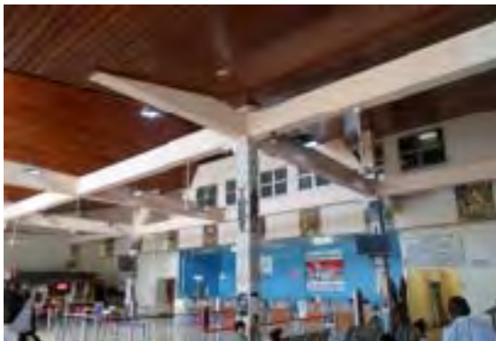
Photo 42 Lights in Check-in Hall
