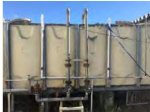
Photo 33 FRP Water Tank
