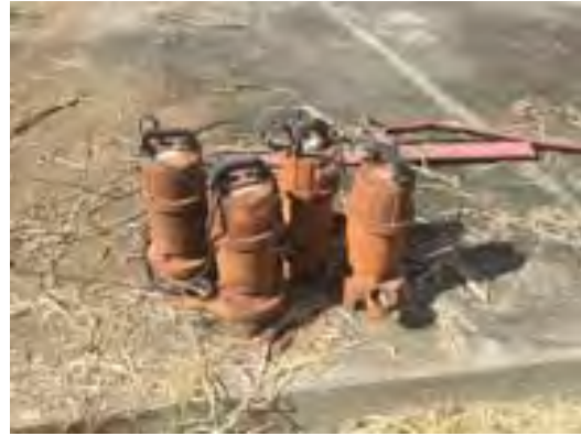
Photo 39 Sewage Water Pump
