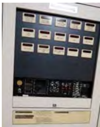
Photo 46 Receiver of Automatic Fire Alarm System
