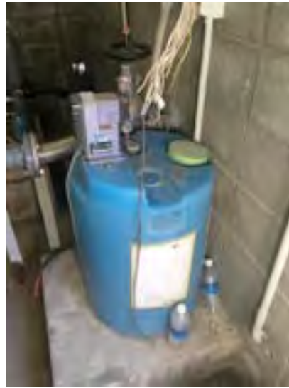
Photo 35 Chlorine Sterilization Unit
