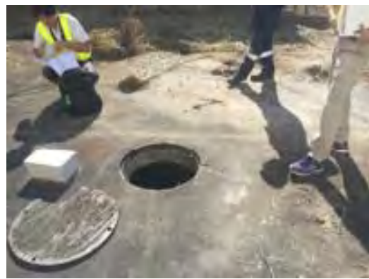
Photo 31 Rain Water Tank and Man Hole
