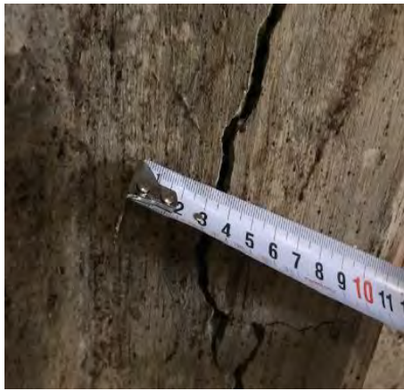
Photo 50 Details View of Crack on a Column of Air Traffic Control Tower
