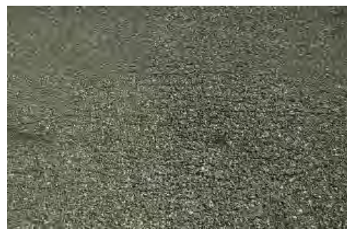
Photo 3 Alligator crack on the International Apron (Unit No. 5)
