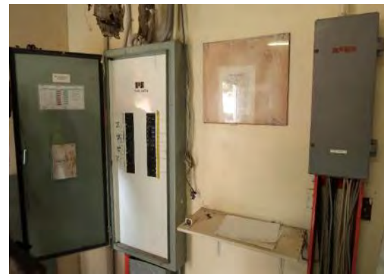
Photo 63 CCR's Distribution Board
