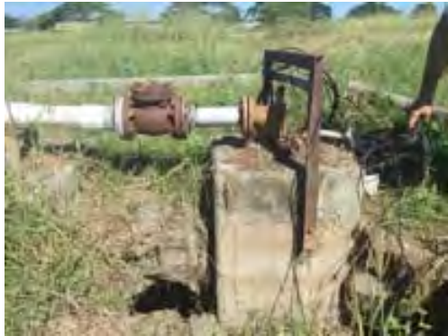
Photo 28 Deep Well Pump
