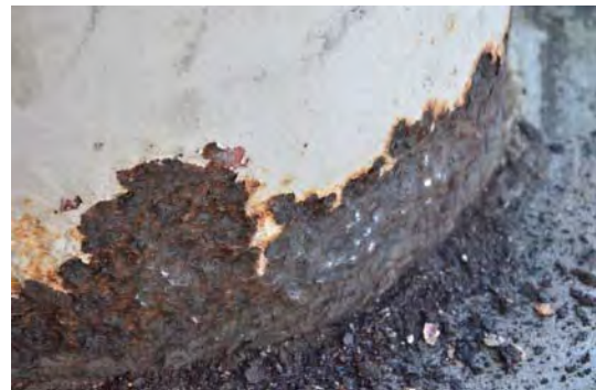
Photo 25 Rust Damage on Column Base at Airside (2)
