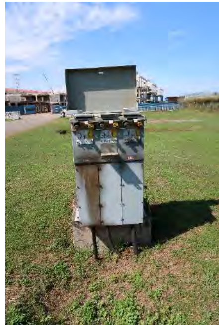
Photo 55 Ring Main Unit
