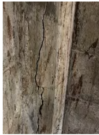
Photo 51 View of Crack
