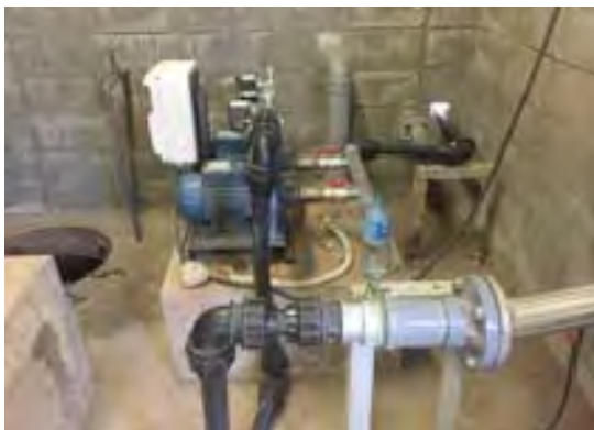
Photo 32 Water Supply Pump Unit
