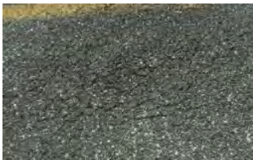
Photo 2 Alligator crack on the International Apron (Unit No. 2)
