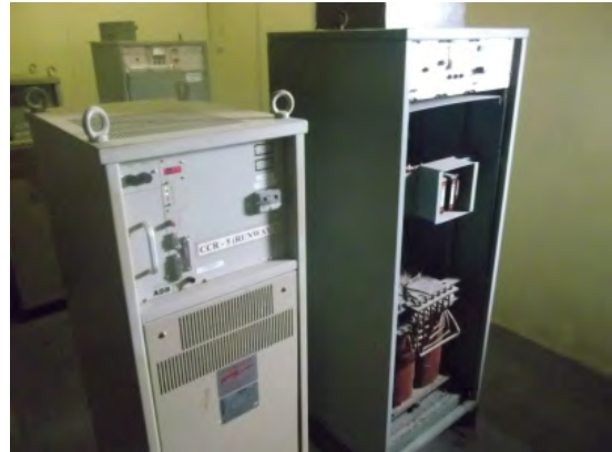
Photo 9 CCRs in the CCR Building
