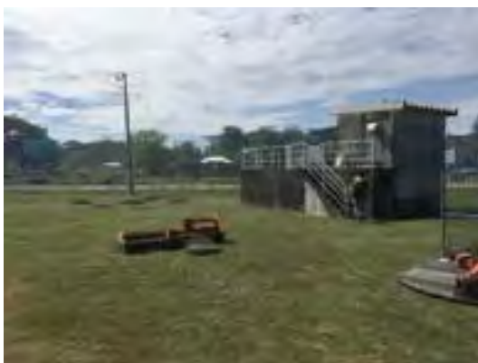
Photo 36 Sewage Treatment Area
