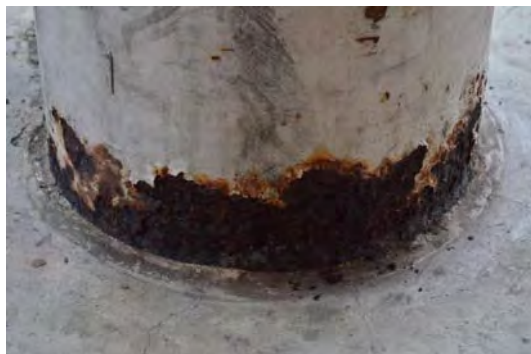
Photo 24 Rust Damage on Column Base at Airside (1)
