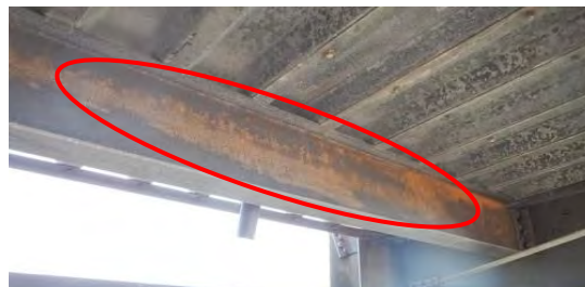
Photo 2.2 Example of Corrosion of Galvanized Coating in Sri Lanka
