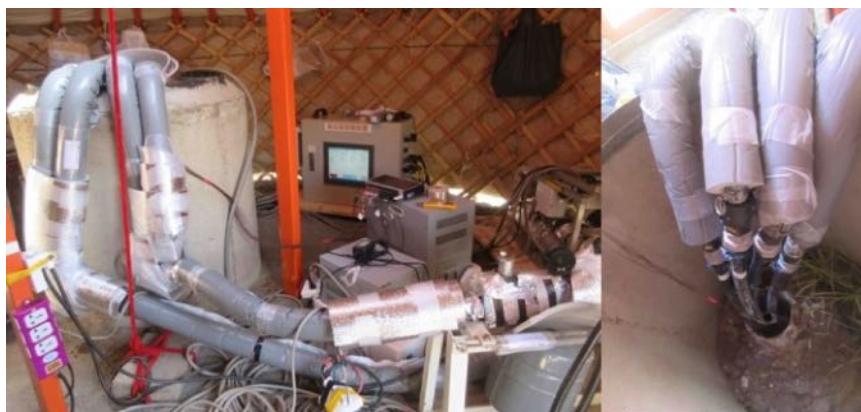
Photo 2 TRT system and well head
