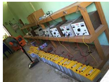
Battery Recharging System
