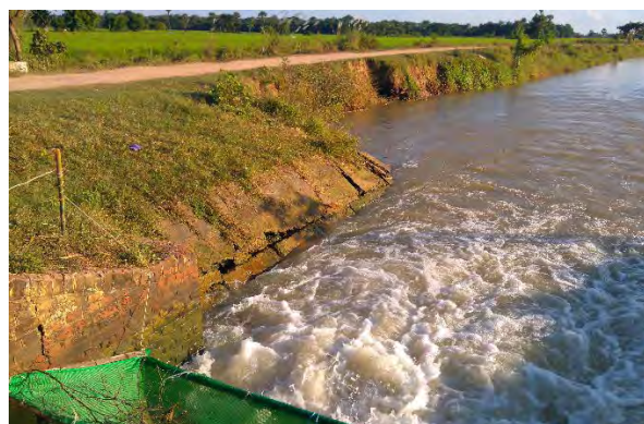
Slope protection at the D/S of the drop structure is damaged and canal at the D/S of slope protection is scoured
