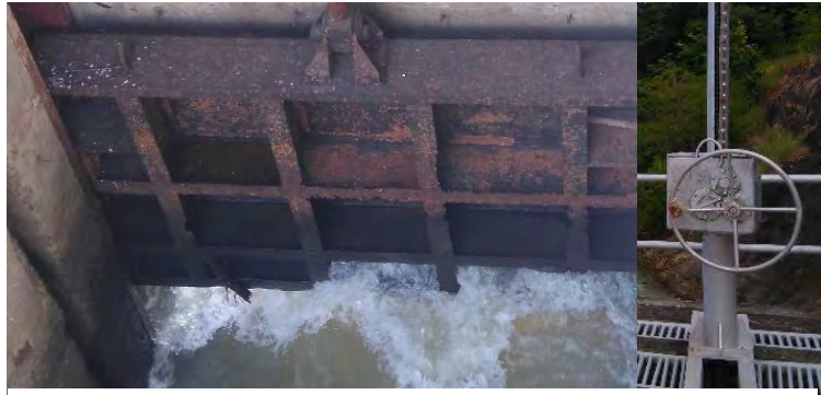
Intake gate for OMC and manual lifting device: the existing plate girder of the gate leaf has been corroded by rust.
