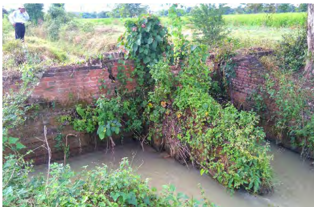
Damaged Drop Structure in Dy23 of YMC: It is an original structure constructed before 1918. It was damaged due to piping.
