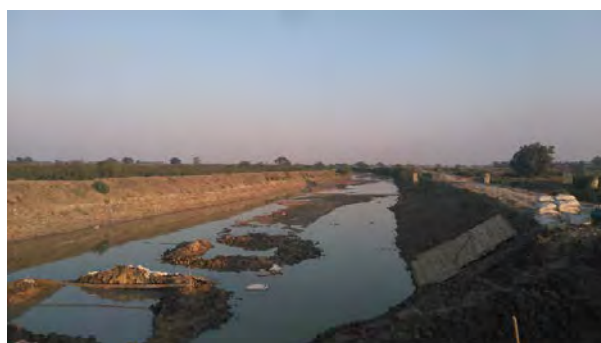
Although expansion of the drainage canal has been continuously implemented by own budget, there are many drainage canals which need to expand the section.
