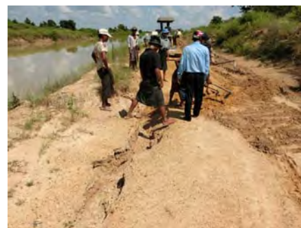
Condition of Canal Maintenance Road after Rain
