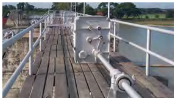
Gate lifting device is a manual operation type. Reducing the operation load, counterweight is installed to balance with gate. There are some aged and damaged portions on the wooden deck.
