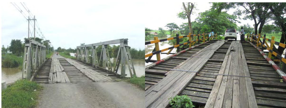
Typical Wooden Bridges in the Project Area, to be improved under the Project
