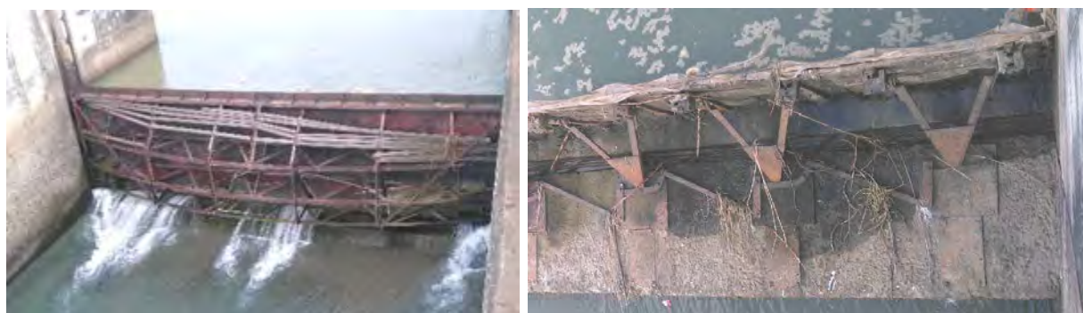
The undersluice gate (upper photo) and shutter gates (lower photo) was installed after damaged by the 1956's largest flood.
