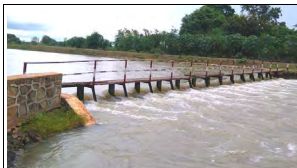
Cross Regulator (Steel frame type)
