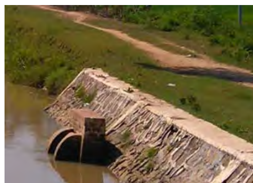
Direct outlet without gate at Branch Canal
