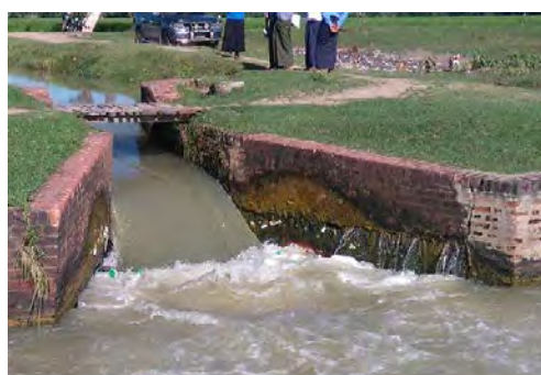
Drop Structure installed at Dy-6 of SMC: It is original structure constructed before 1905. There is leakage through cracks on the wall.
