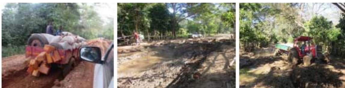
Phot. 5 Unpaved road condition between Ambanja and the Upstream site
