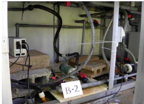
Tank B : Circulation system was aging
