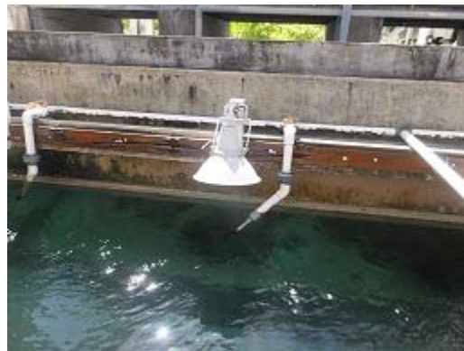
Lighting fixture for tank G
