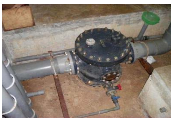
Strainer for intake pump: Good condition
