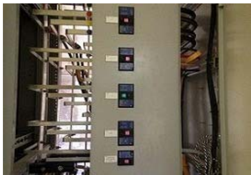
Main distribution board
