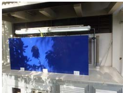
Lighting fixture for tank B
