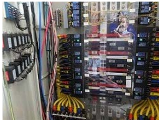
P-2 Distribution board in Aquarium
