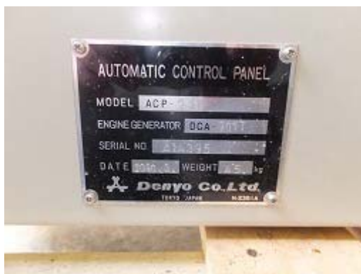
Nameplate of automatic control panel
