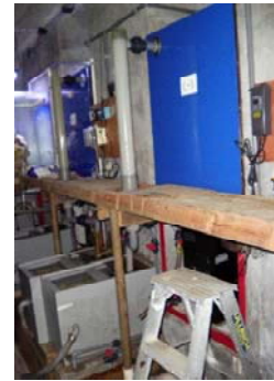
Tank C : Circulation system was aging
