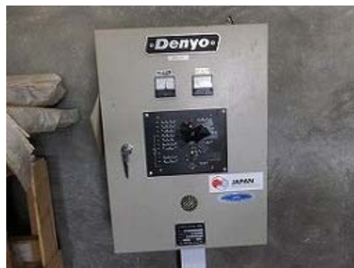
Existing automatic control panel
