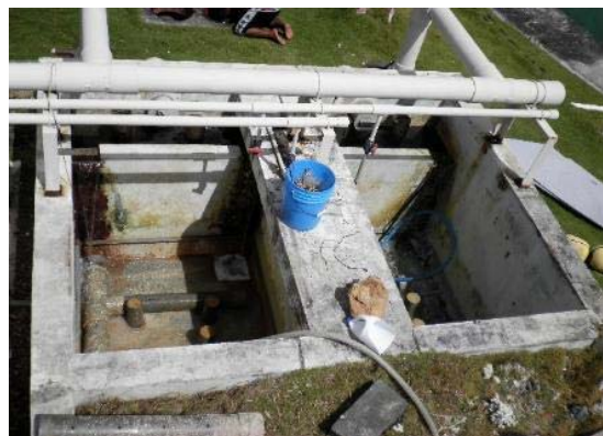
Filter tank for tank N and G : No function
