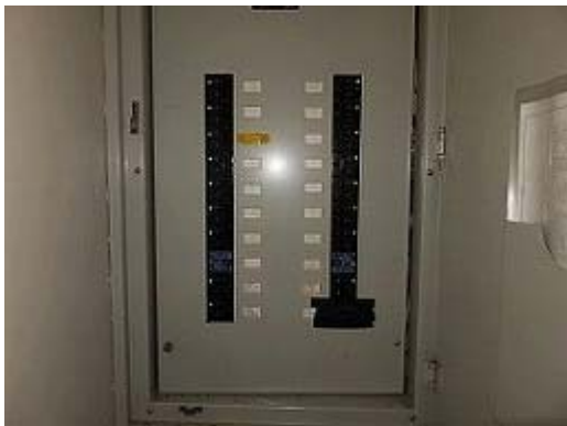
L-1 Distribution board in Research bldg.
