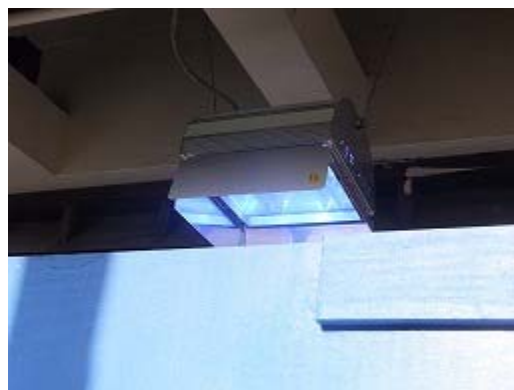
Lighting fixture for tank H
