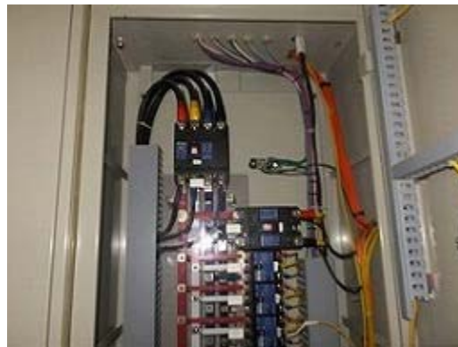
P-1 Distribution board in Research bldg.
