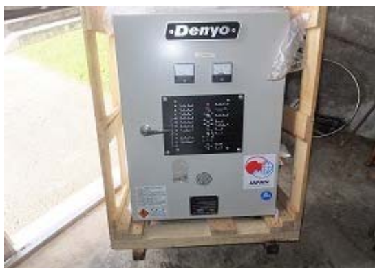
Automatic control panel
