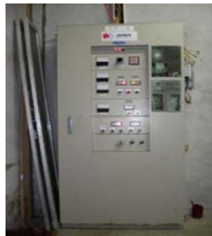
Control panel of seawater intake :Good
