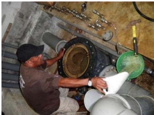
Cleaning maintenance of strainer
