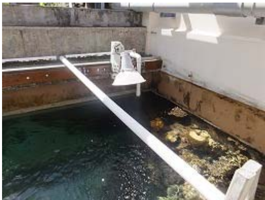
Lighting fixture for tank G
