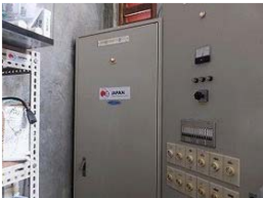
L-2 Distribution board in Aquarium
