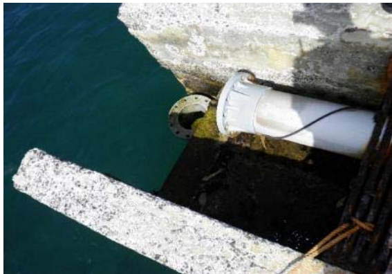
Old intake pipe: Not functioning
