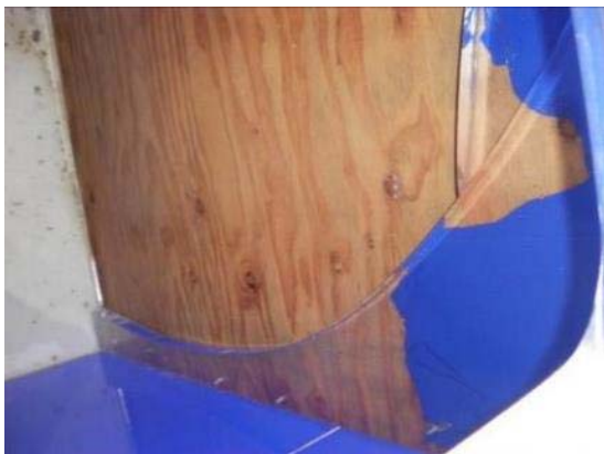
Tank H : Corruption of tank back board
