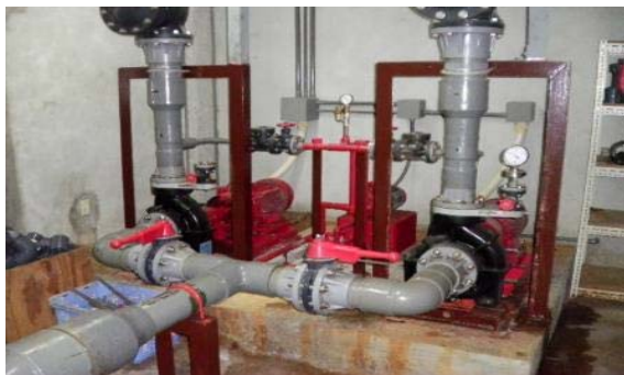
Seawater intake pumps : Good maintenance
