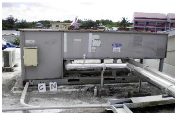
Water chiller for tank N and G :No function
