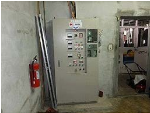
CP-A Distribution board in Research bldg.
