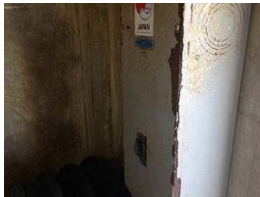
Switch gear for Annex bldg.
