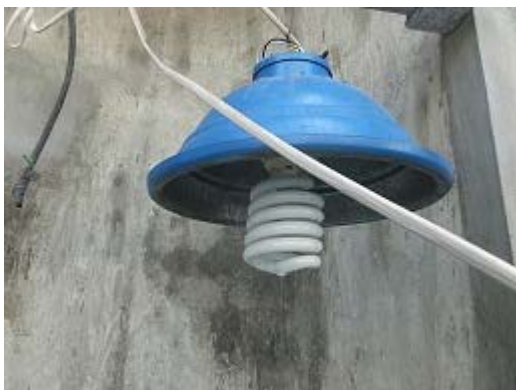
Lighting fixture for tank O
