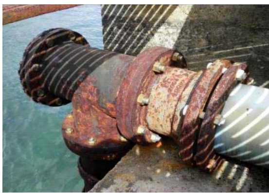
Existing intake pipe : Rust corrosion of steel
