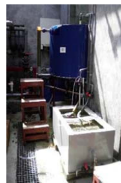
Tank O : Circulation system was aging
