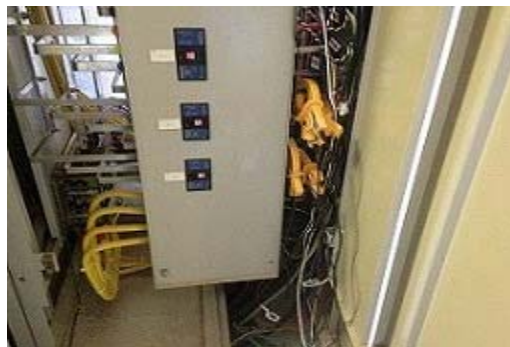
Main distribution board
