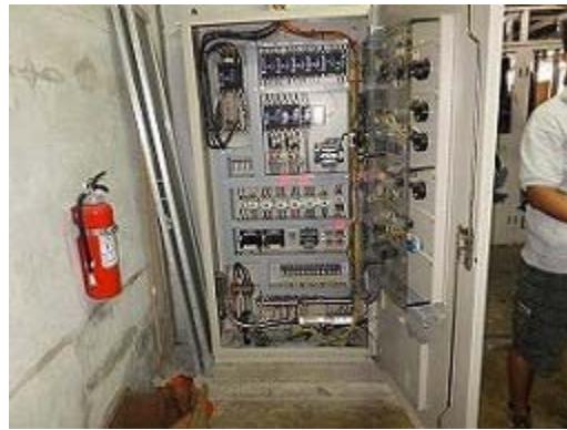
CP-A Distribution board in Research bldg.
