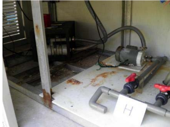
Tank H : Circulation system was aging
