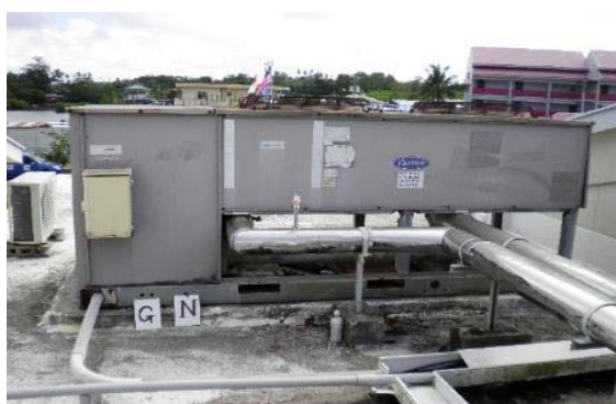
Water chiller for tank N and G :No function
