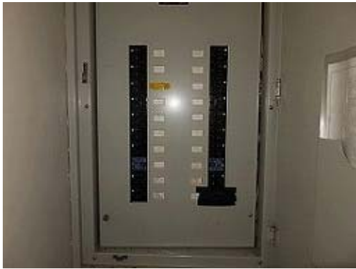
L-1 Distribution board in Research bldg.
