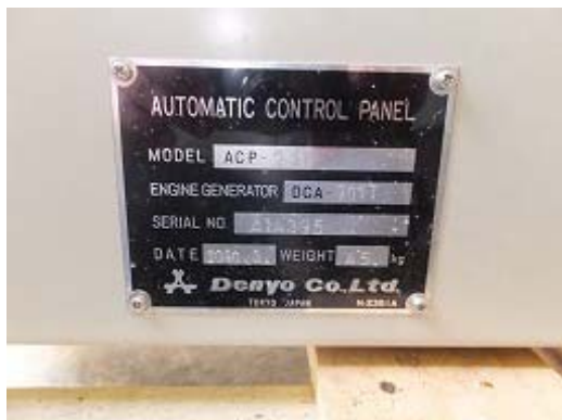
Nameplate of automatic control panel
