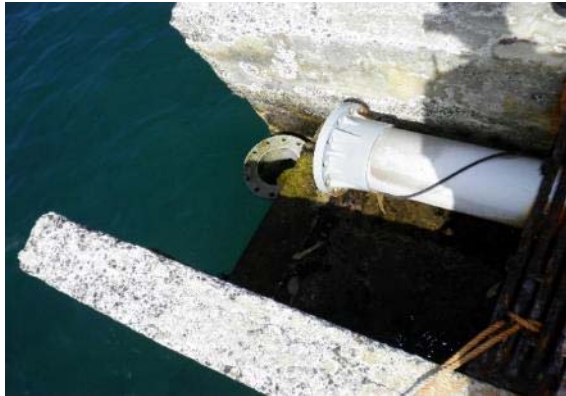
Old intake pipe: Not functioning
