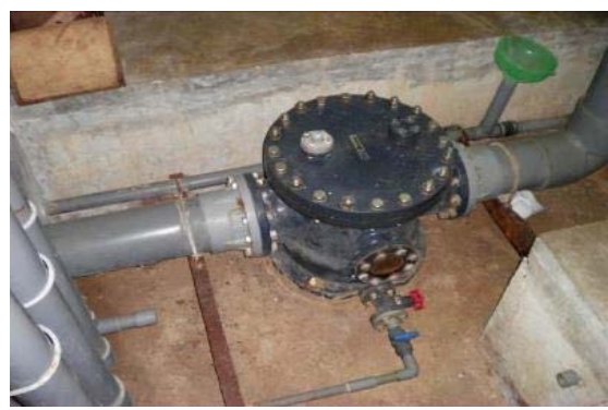
Strainer for intake pump: Good condition
