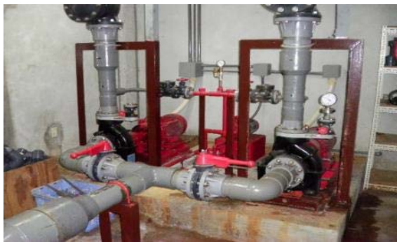
Seawater intake pumps : Good maintenance
