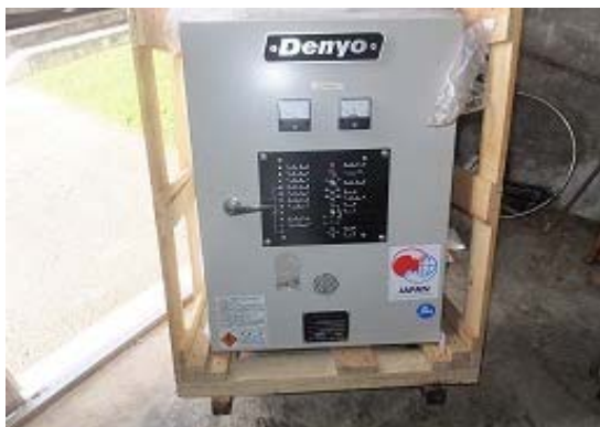
Automatic control panel
