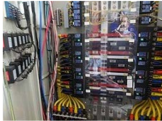
P-2 Distribution board in Aquarium
