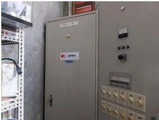
L-2 Distribution board in Aquarium
