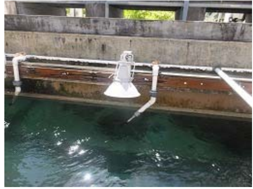
Lighting fixture for tank G
