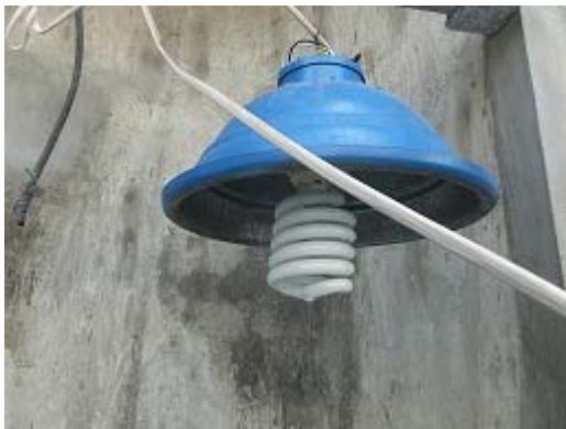
Lighting fixture for tank O
