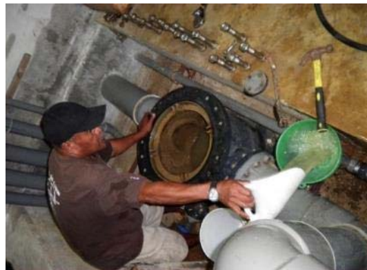
Cleaning maintenance of strainer
