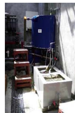
Tank O : Circulation system was aging
