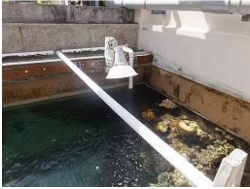
Lighting fixture for tank G
