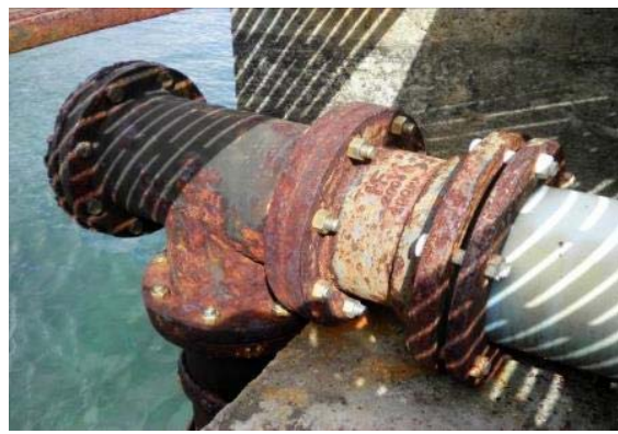
Existing intake pipe : Rust corrosion of steel
