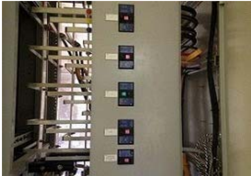
Main distribution board
