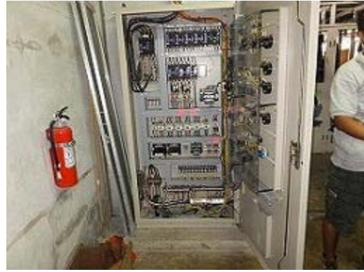
CP-A Distribution board in Research bldg.
