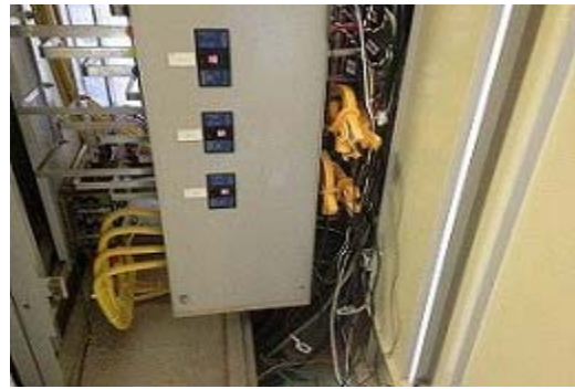
Main distribution board
