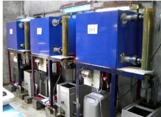
Tank D : Circulation system was aging
