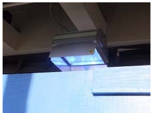
Lighting fixture for tank H
