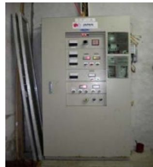
Control panel of seawater intake :Good
