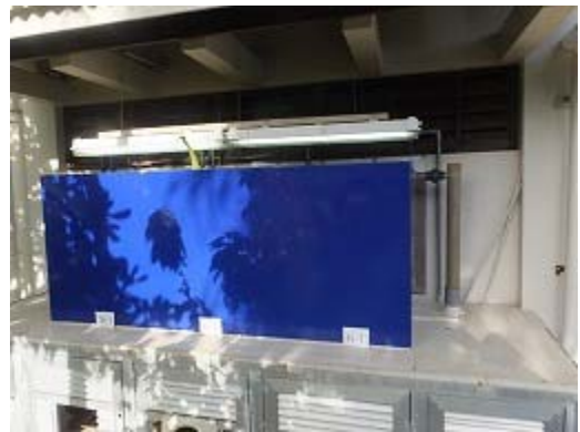
Lighting fixture for tank B
