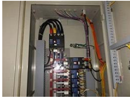
P-1 Distribution board in Research bldg.
