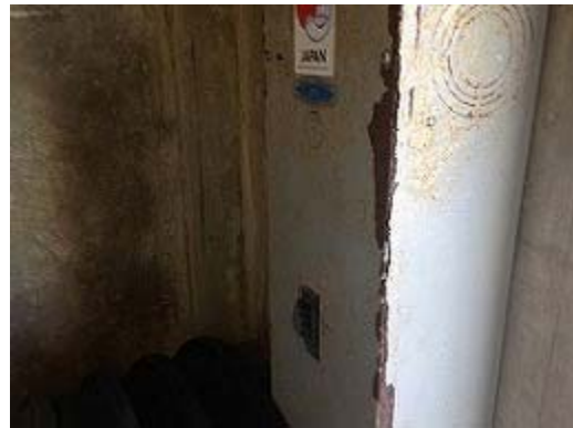
Switch gear for Annex bldg.
