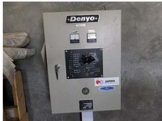
Existing automatic control panel
