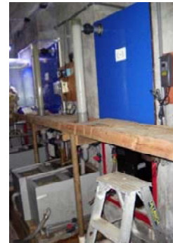
Tank C : Circulation system was aging
