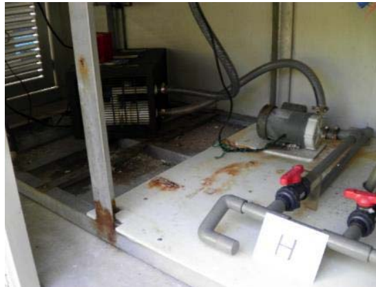
Tank H : Circulation system was aging
