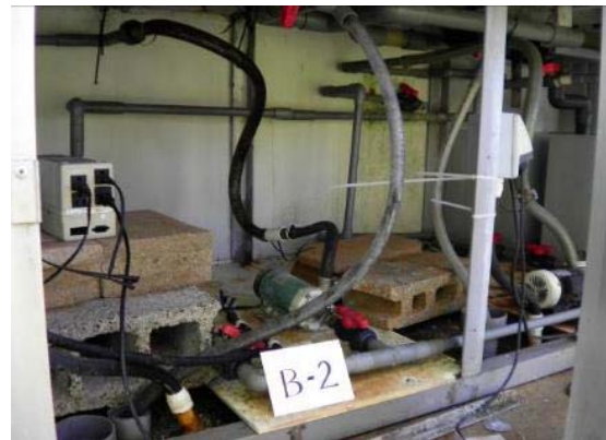
Tank B : Circulation system was aging
