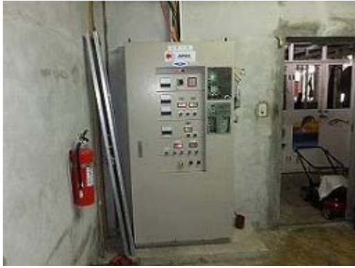
CP-A Distribution board in Research bldg.
