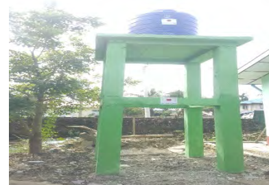
Water System January 2018
