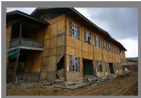
Cyclone Komen destroyed hundreds of school buildings..
