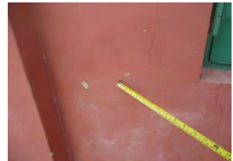
3-4c Defect of plaster cracking to corner of window
