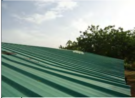
2-8 Roofing damage by wind due to fixing defect
