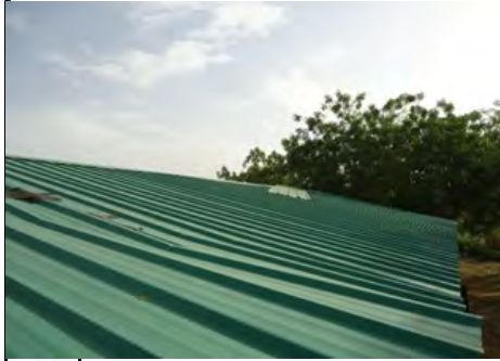
2-8 Roofing damage by wind due to fixing defect
