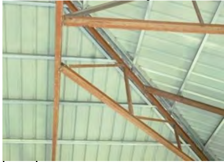
2-7c No rust proof paint to steel trusses
