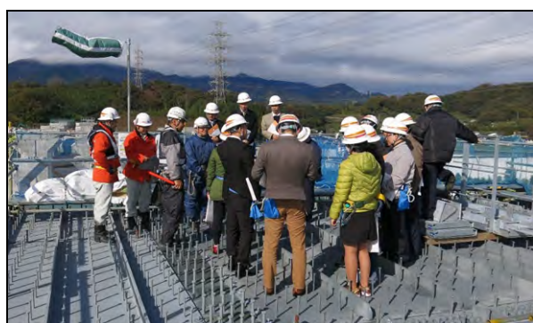
Site visit (S3) / 26 Nov. 2015 New Tomei Expressway (Isehara City, Kanagawa Pref.) Central Nippon Expressway Co. Ltd.
