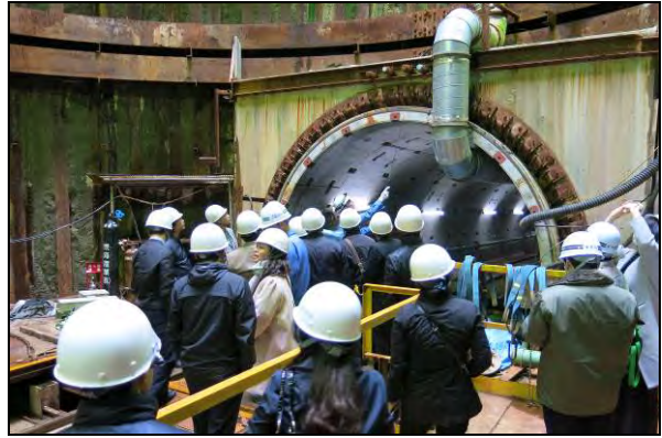
Site visit (S6) / 16 Nov. 2016 Shin-Isogo Sewer Pipe (Construction Site) (Yokohama City, Kanagawa Pref.) Yokohama City
