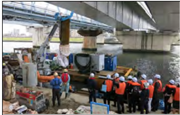
Site visit (S1) / 18 Nov. 2015 Bank reconstruction (Edogawa Ward, Tokyo) Arakawa-Karyu River Office Kanto Regional Development Bureau, MLIT,
