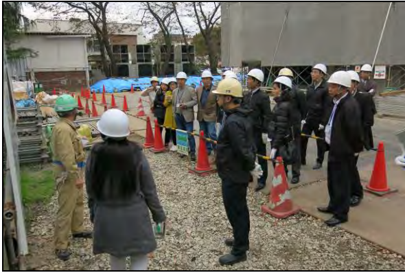
Site visit (S5) / 16 Nov. 2016 Asaka Public Employment Security Office Building (Construction Site) (Asaka City, Saitama Pref.) Government Building Planning Division Kanto Regional Development Bureau, MLIT & Tokyo Government Building Office-1 Kanto Regional Development Bureau, MLIT
