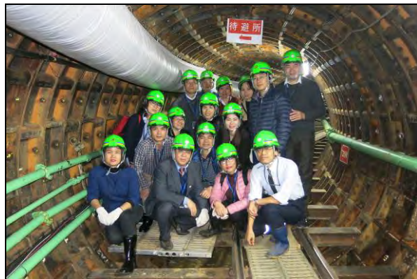
Site visit (S4) / 01 March 2018 Storm sewer (Construction Site) (Yokohama City, Kanagawa Pref.) Yokohama City
