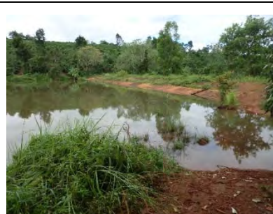
Fig 4. Dak Ri Reservoir (erthfill dam, capacity=0.375MCM, dam crest length=88 m) constructed by DPC and operation by farmers. In the 2015/16 drought, the reservoir was mostly dried up.
