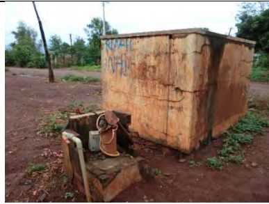
Fig 1. Old domestic water supply for Ia Blu Commune using a deep well (Depth=80 m, D=145 mm) was built by DPC in 1992. The strainer of the well is clogged in 2017 and it no longer can be used.
