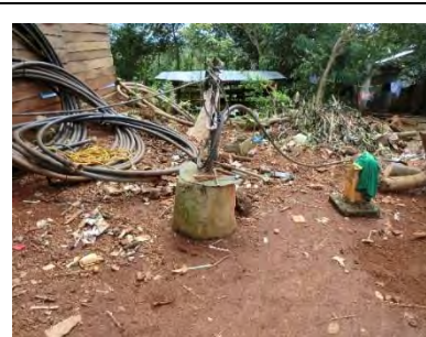
Fig 6. Deep well for domestic water (Depth=90 m, D=100 smm). It took 2 months to recover the GWL after the drought in 2015/16.
