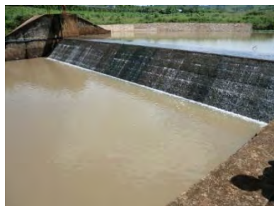
Fig 4. Ia Ke irrigation weir (W=20 m, H=2.65 m, Q=about 1.0 m 3 /s) supply water for 25 ha of paddy field constructed by DPC in 2007. In the 2015/16 drought, the river water was mostly dried up. There is no regulation and operation record.
