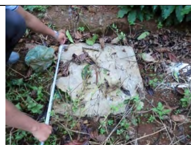
Fig 3. Deep well for irrigation of coffee and pepper (Depth=80 m, D=90 mm).
