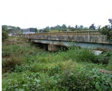
Fig 4. The national road bridge in the upstream of the Cau Xanh River
