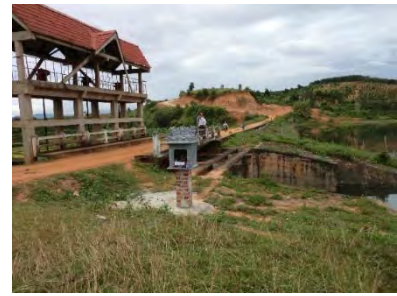
Fig 6. Control gate of Dak Trit Reservoir (upstream of the inundated area)
