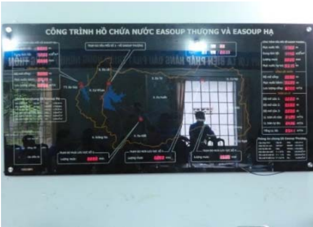
Real time telemetric meteo-hydrological monitoring system installed by MARD Pilot Project in 2010 (District: Ea Sup, Commune: Ya To Mot)
