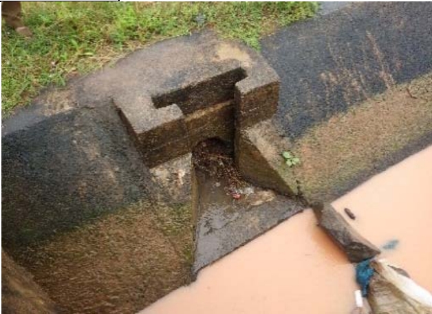
The gate was stolen and the canal got stuck due to an ineffective O&M activity (District: Ea Sup, Commune: Ya To Mot)
