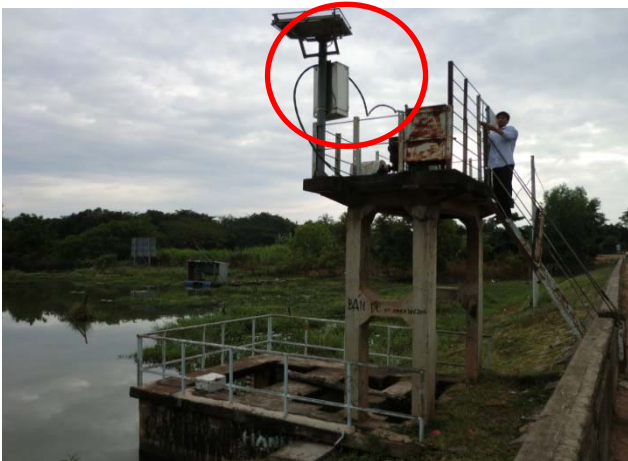
Telemetric rainfall and reservoir water level monitoring system (District: Ea Sup, Commune: Ya To Mot)
