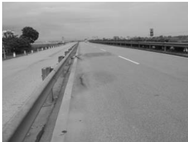
Image 5.5.17 Depression on asphalt pavement
