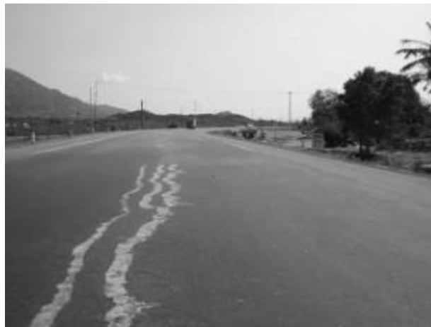
Image 5.5.1 Bleeding and fatting-up of asphalt pavement
