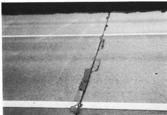
Image 5.6.7 Lost edges at the joint edge (repaired by resin mortar)
