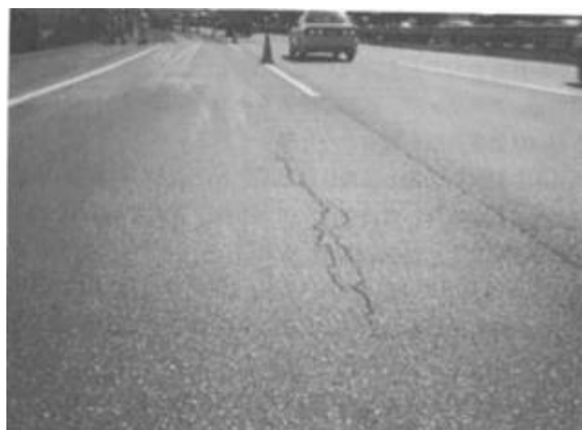
Image 5.5.8 Longitudinal single crack
