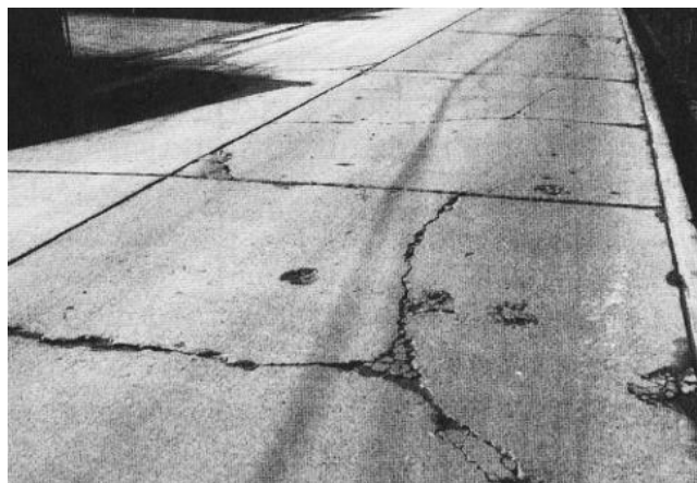
Image 5.6.11 Tortoise shell crack
