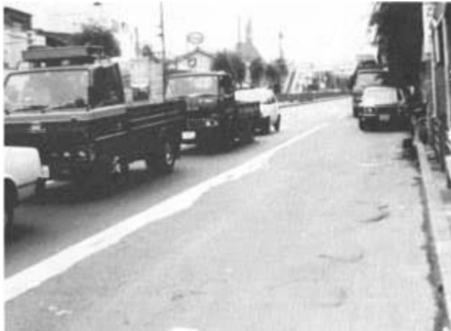
Image 5.5.16 Shoving of asphalt pavement
