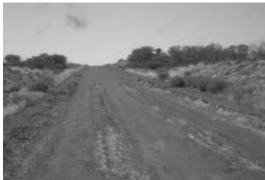
Image 5.5.3 Raveling of asphalt pavement
