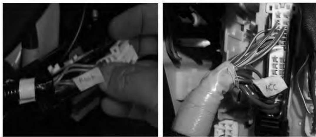
Figure 12.35 Stick labels for the cables
