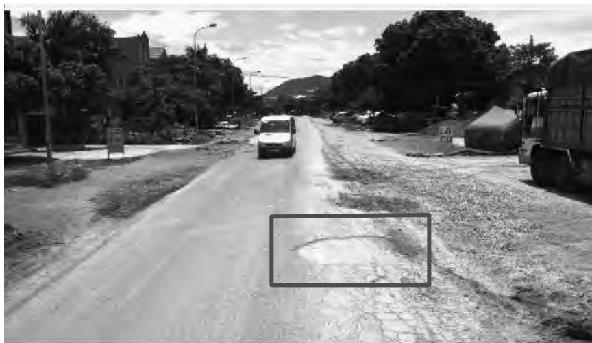
Figure 9.47 Pothole – Forward View
