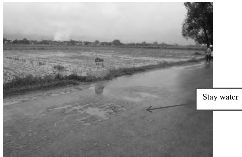
Figure 3.22 Road conditions where survey cannot be restarted (sample-1)
