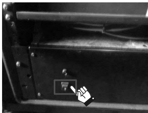
Main control unit
