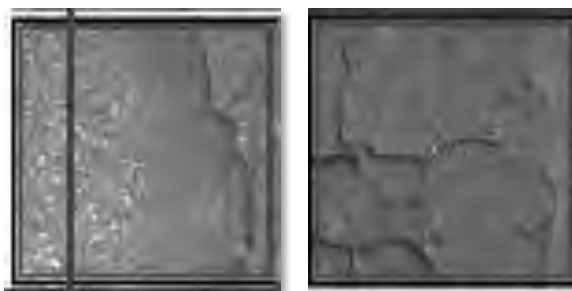
Figure 9.45 Two or More Crack
