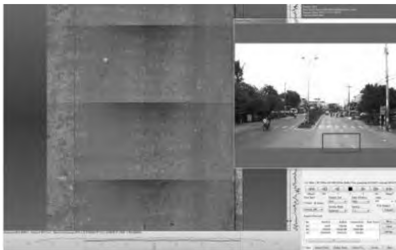
Figure 4.10 Example of visible the crack only forward view image
