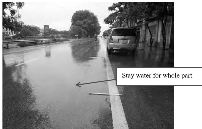
Figure 3.23 Road conditions where survey cannot be restarted (sample-2)
