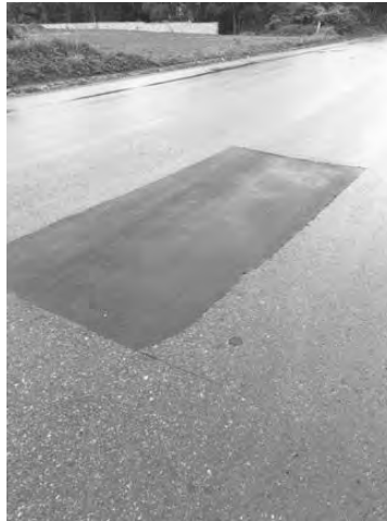
Photo 6.1-15 Damage condition on site 09
