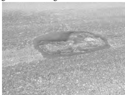
Photo 6.1-13 Damage condition on site 06
