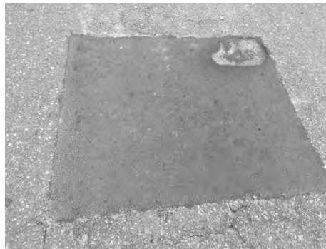
Photo 6.1-12 Damage condition on site 05
