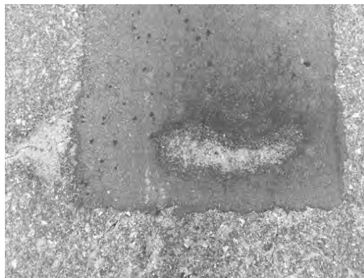
Photo 6.1-16 Damage condition on site 10
