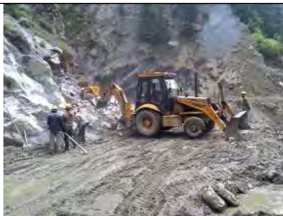
Road Blocked due to the Land Slide on the way from Pangti, Chmaba District to Udaipur, Lahaul & Spiti District (14 June 2017)
