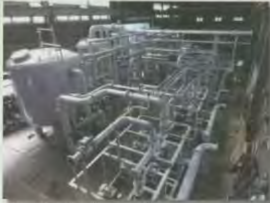
The water treatment system implemented by Tokai.
